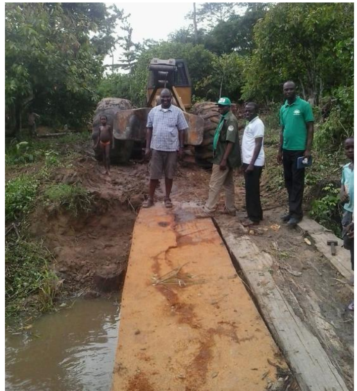
Timber right holder repairing Aboaboso bridge after meeting with all committee members in a group.
